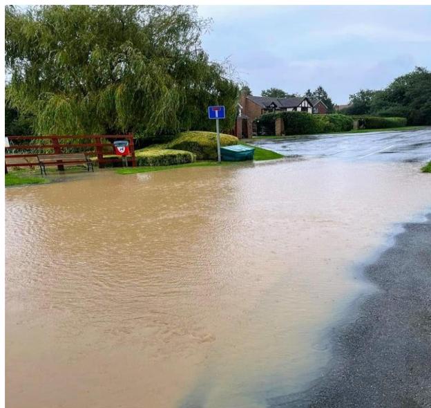
Peppin Lane and Louth Road junction showing overflowing 'Dock' covering the entire road width and beyond. Fed from culvert and attenuation chamber near A16 Short Lane (Storm Babet Oct 23)
